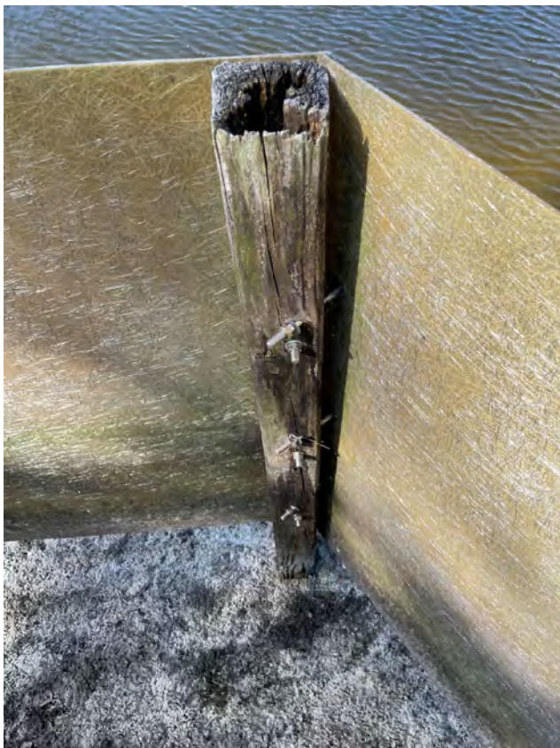
Deteriorating wood at Pond T2 weir outfall
