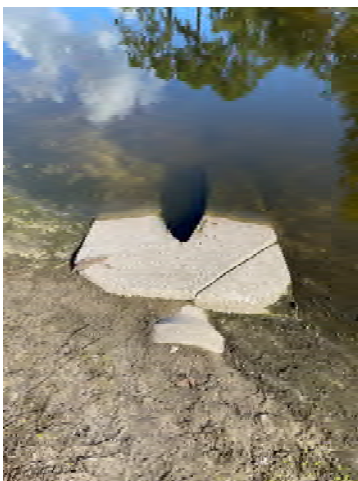
Minor crack in 18" MES at Pond T2
